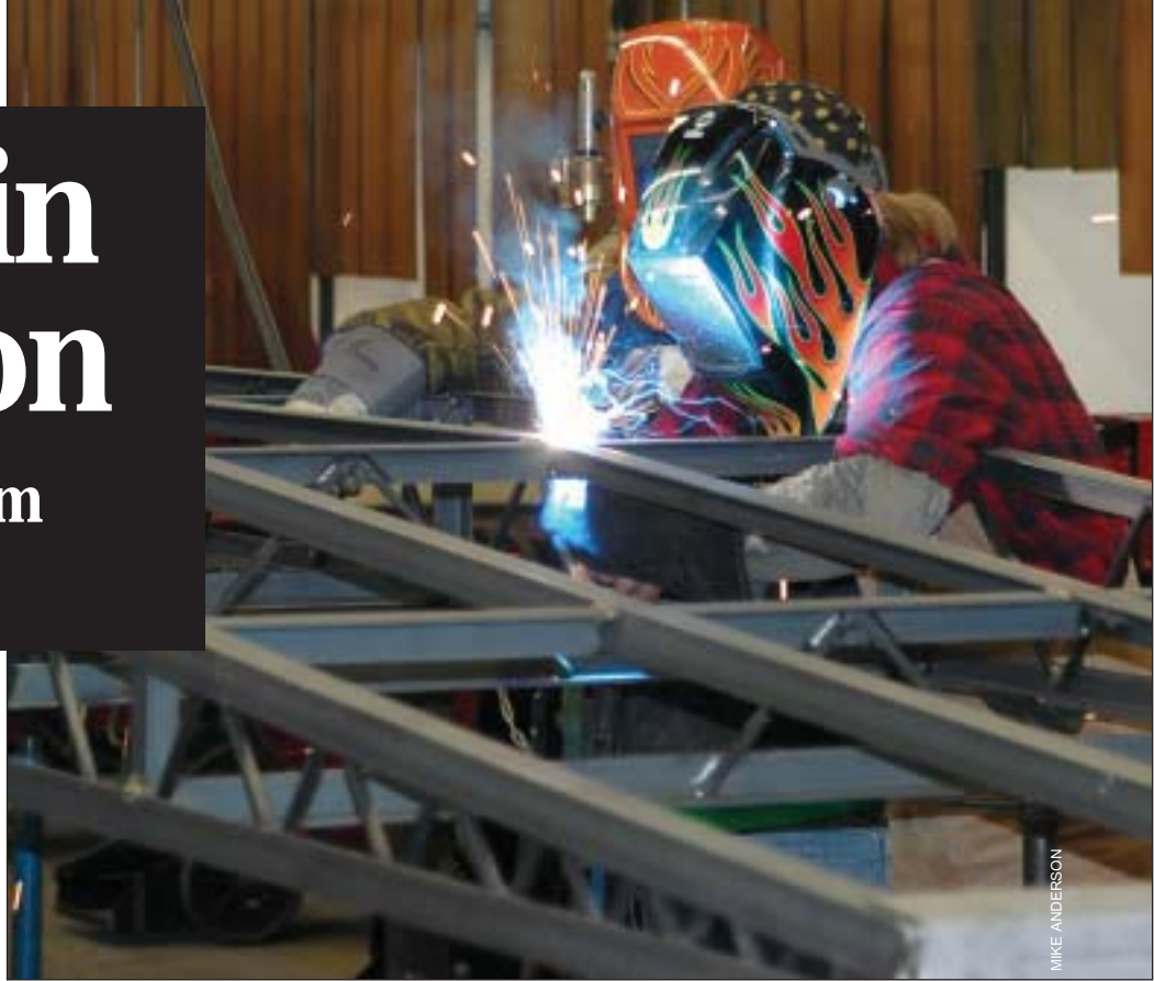
North Dakota State College of Science students weld one of several courtesy docks expected to be constructed at the college in Wahpeton this year.
