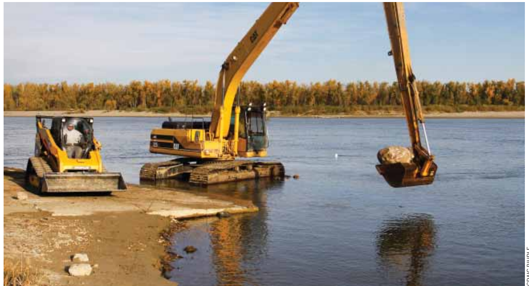
Work on the Sugarloaf boat ramp on the Missouri River south of Mandan. By the time construction season ended, only one ramp on the Missouri was still unusable because of flood damage that occurred in 2011.
