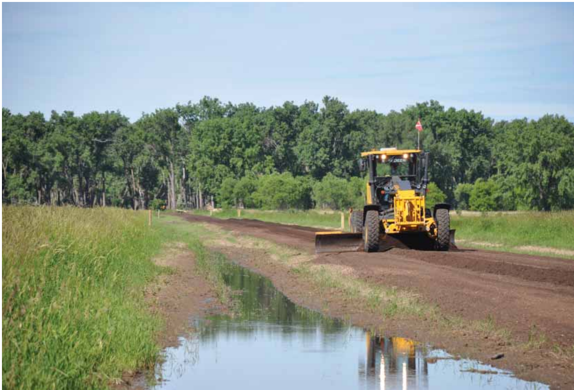
The Game and Fish Department, in cooperation with Burleigh County, tackled major road repairs earlier this summer on Oahe WMA south of Bismarck. The project included reshaping and graveling about 8 miles of access roads at MacLean Bottoms and Apple Creek.
