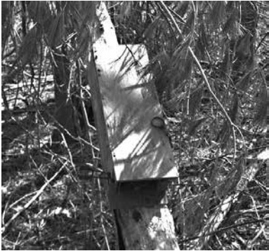
Leaning pole set.
